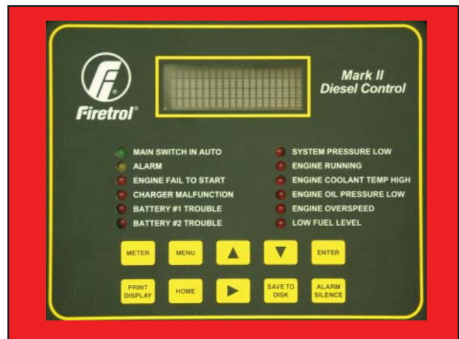
Door mounted display/interface panel
