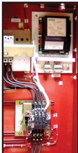
FTA975 Isolating Switch, ASCO Transfer Switch and Control Panel
